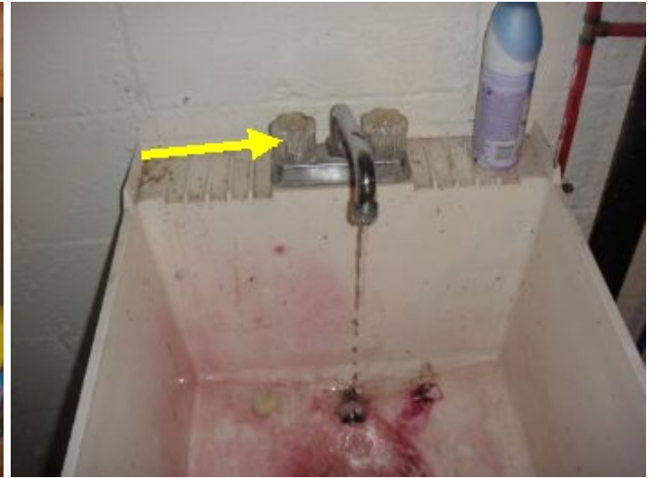
Laundry Wash Basin
