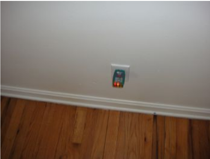
Master Bedroom Electrical
