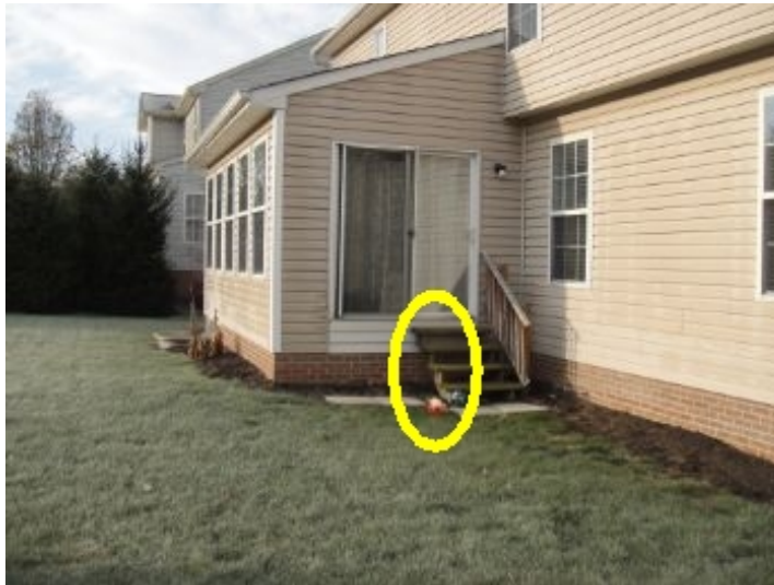
Missing handrails and balusters.
