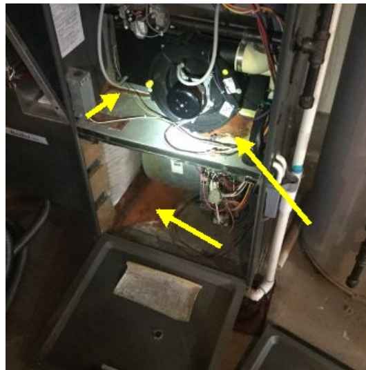
Rust and flaking observed
