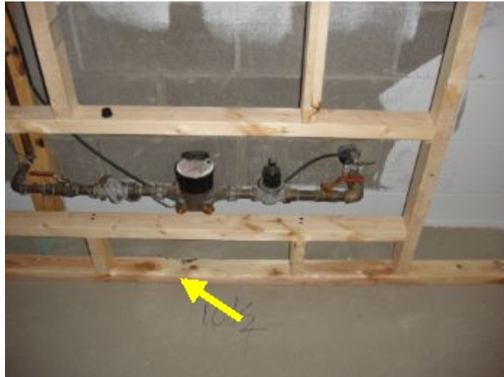
Bare wood in touch with masonry needs to be treated
