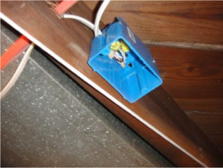
Basement/Crawlspace Basement Electric
