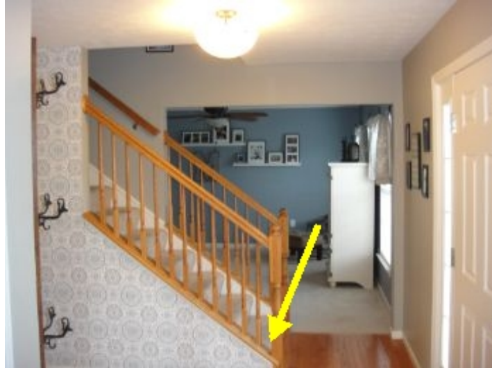
Loose hand rail on left side needs secured
